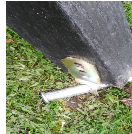
A bracket completely destroyed
